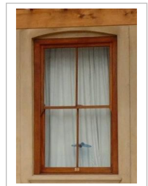
Figure 10: Vertically proportioned window with plastered windowsill and simple plaster-band forming a flat arch above the window.
